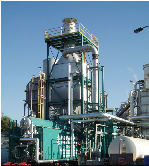
A CataStak™ SCR system helped a paper mill in California reduce GHG emissions. The 120,000 lb/hr, 175 psi boiler operated at 5 ppm NOx and easily meet local air quality requirements.
